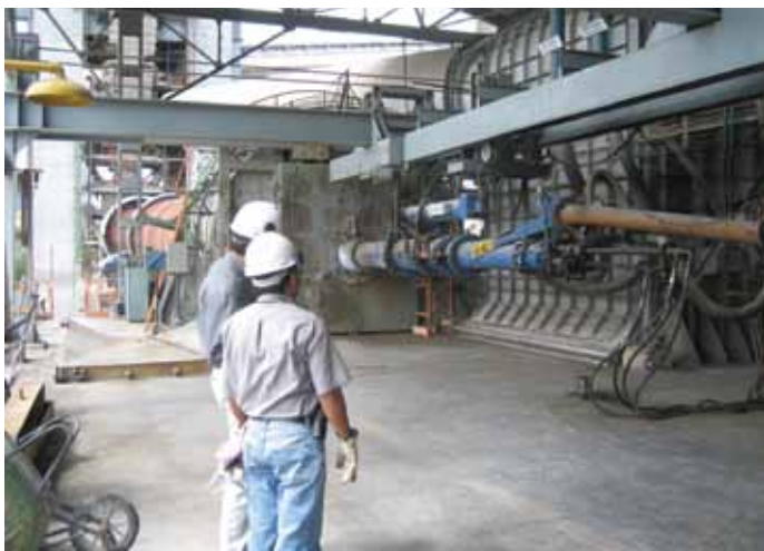
Figure XX.1: feeding of liquid and pulverised waste through the main burner
